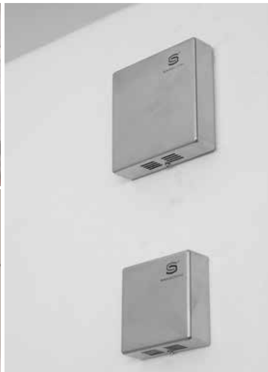
Oberer Sensor: CO 2 -Sensor
